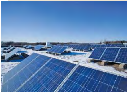
Photo voltaic panels provide active solar energy generation.
